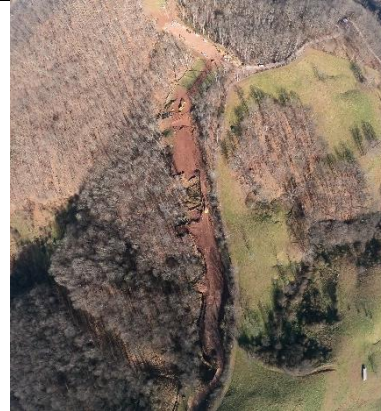
Milepost 46.6 G0024928.jpg Construction underway. Large bare, unvegetated areas. Sediment flowing into stream crossings. Slip occurring on north side of photo.
