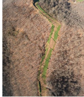
Milepost 60.8 G0024671.jpg Several areas with lack of vegetation on steep slopes.
