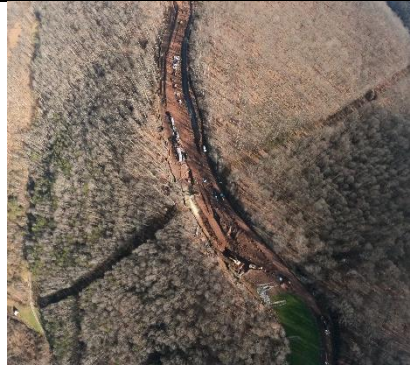
Milepost 57.3 G0024732.jpg Construction underway at what appears to be an interconnect point.
