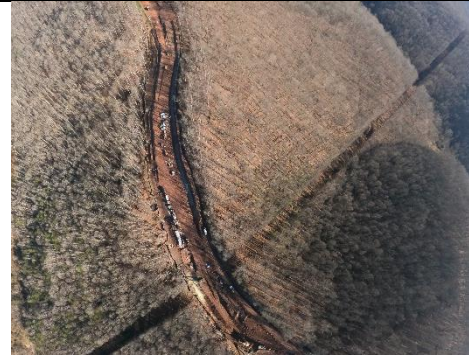
Milepost 57.2 G0024733.jpg Large areas of bare dirt. There is no vegetation in ROW. Area under construction.
