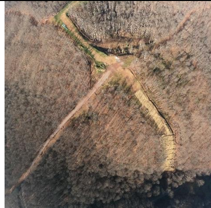
Milepost 59.7 G0024690.jpg Bare areas at and near intersection with extremely steep access road.
