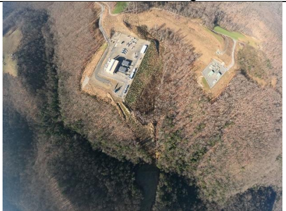
Milepost 77.5 G0024358.jpg Rock/dirt piles/sediment coming off of hillside and slope around Compressor station
