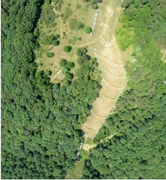
Milepost 188.8 Seeding needed on slope above stream crossing.
