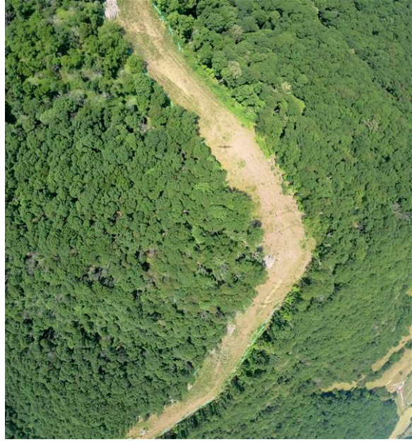
Milepost 189.3 Exposed soil on slope needs additional seeding.
