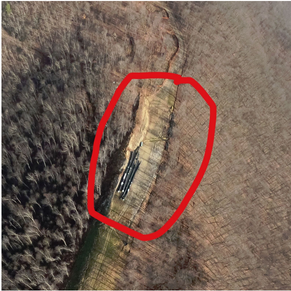
Milepost 95.6 G0024052.jpg Bare area with pipe lying on ground, Very little vegetation in ROW. Seeding required.
