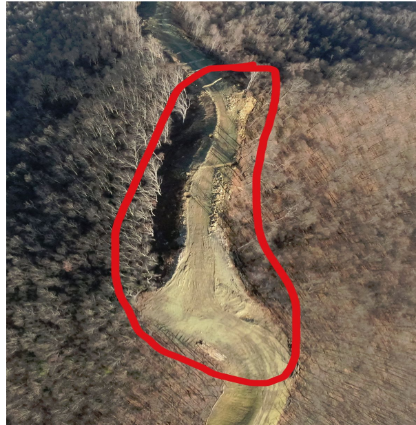
Milepost 84.7 G0024239.jpg This area has sparse vegetation. It has lain bare for more than 6 months. Very remote location. Inspection requested.
