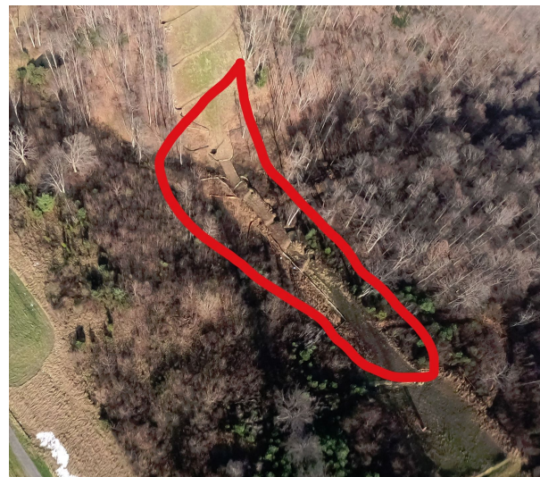
Milepost 80.8 G0024302.jpg Bare areas on both sides of stream crossing. Inspection requested.
