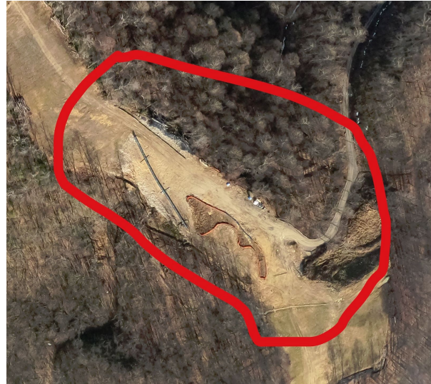
Milepost 95.4 G0024059.jpg Large bare area at intersection with access road. Seeding required. There appears to be a slip above the road intersection. Possible sediment flowing off site.
