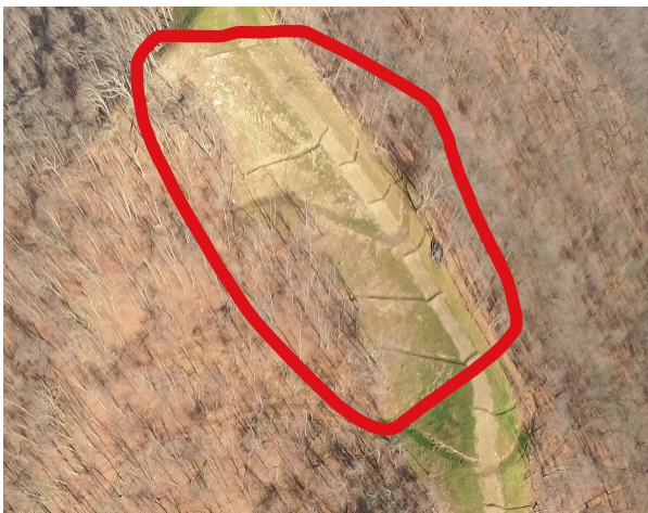
Milepost 83.7 G0024252.jpg Bare areas on the upper slope need reseeding. Inspection requested.
