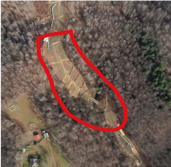
Milepost 109.5 G0023800.jpg The Steep Slope above stream crossing has little vegetation. Waterbars are in need of stabilization and maintenance.
