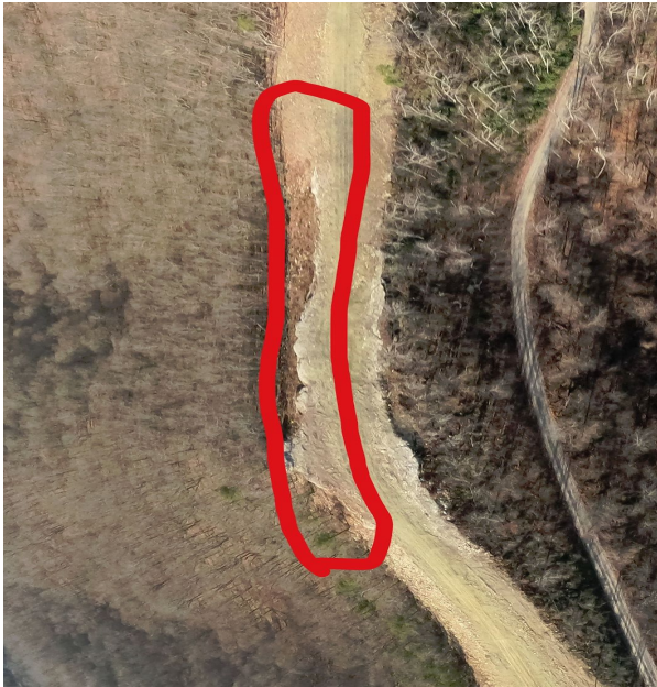
Milepost 86.0 G0024217.jpg Large bare area forming. Soil collapse on slope. Need inspection for stabilization.
