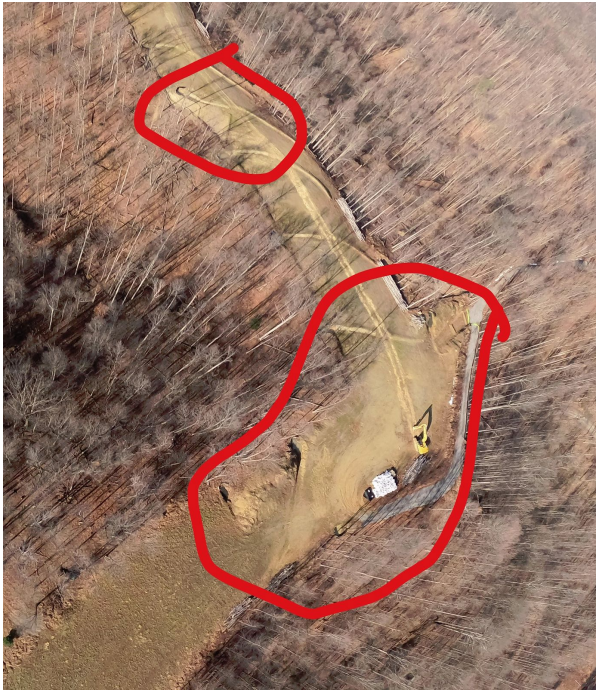
Milepost 80.3 G0024310.jpg Stabilization measures for bare areas are needed. Inspection for cover requested.
