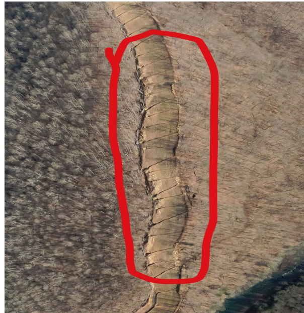
Milepost 87.1 G0024196.jpg Remote area with long steep slope showing signs of erosion. This area needs inspection.
