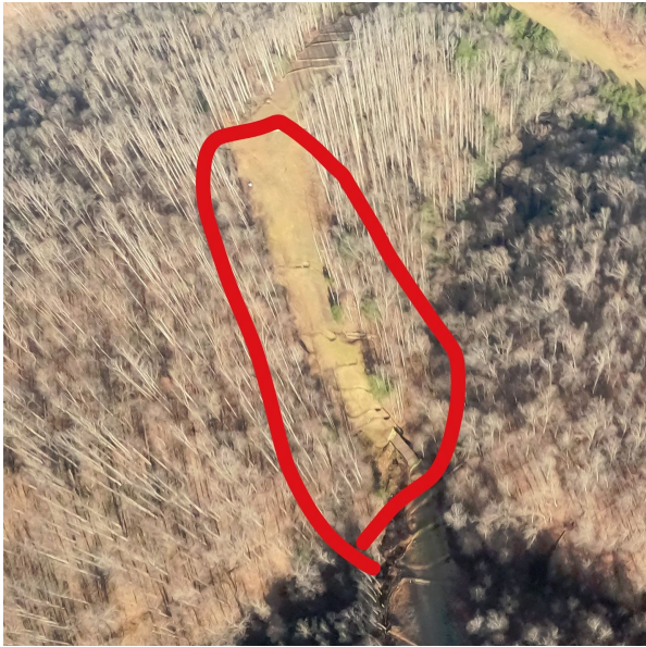
Milepost 82.6 G0024271.jpg Steep slope with sparse vegetation in remote area. Additional stabilization measures needed. Inspection requested.
