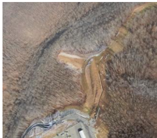
Milepost 154.4 G0023017.jpg Bare or sparse vegetation north of the compressor station site. Re-seeding and maintenance of erosion control devices is needed.
