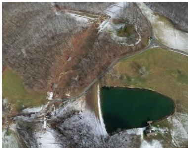
Milepost 148.2 G0023130.jpg Bare/sparsely vegetated areas with rill erosion at toe of slope. Re-seeding required to stabilize slopes.
