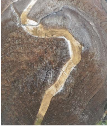
Milepost 143.2 - 143.5 G0023215.jpg Long slope with bare/sparsely vegetated areas and rill erosion. Re-seeding and erosion control matting required to stabilize slopes.
