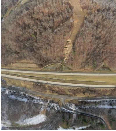
Milepost 156.6 - 156.7 G0022979.jpg Large area with no vegetative cover on steep slope with slips and gullies forming on slope.
