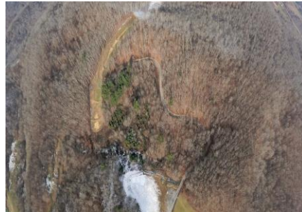
Milepost 155.5 G0022998.jpg Sparse vegetation or dead grass with bare areas and rill erosion at toe of slope.
