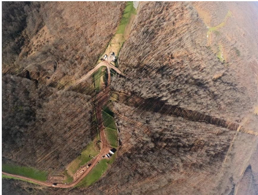
December 2020 flight photo of milepost 56.7 slip location
