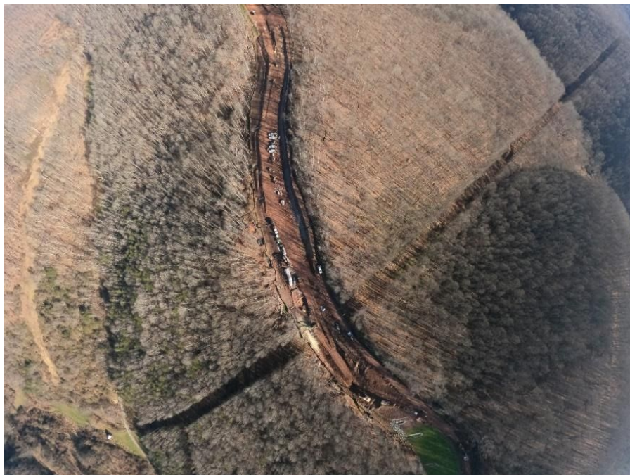
December 2020 flight photo of milepost 57.2 slip location
