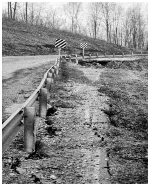
Lewis County, WV Road damage caused by slippage in an area with Gilpin-Upshur silt loam, 35 to 70 percent slope 4
