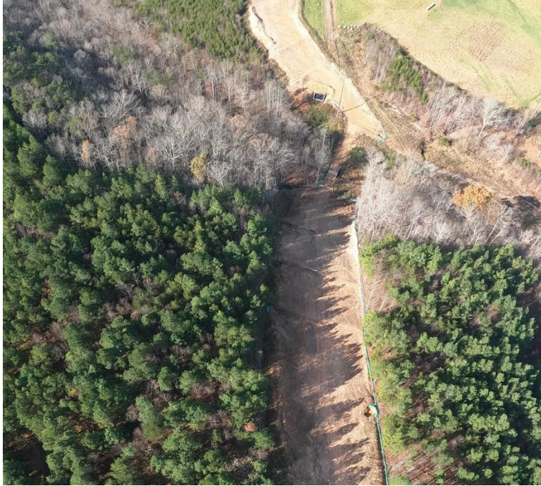
Milepost 283 above Parrott Branch shows areas that are bare or lack vegetative cover.
