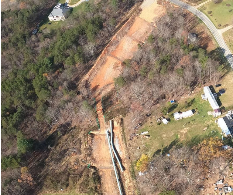
Milepost 271.3 below Golden View Road shows several bare areas with sparse or dead vegetation.
