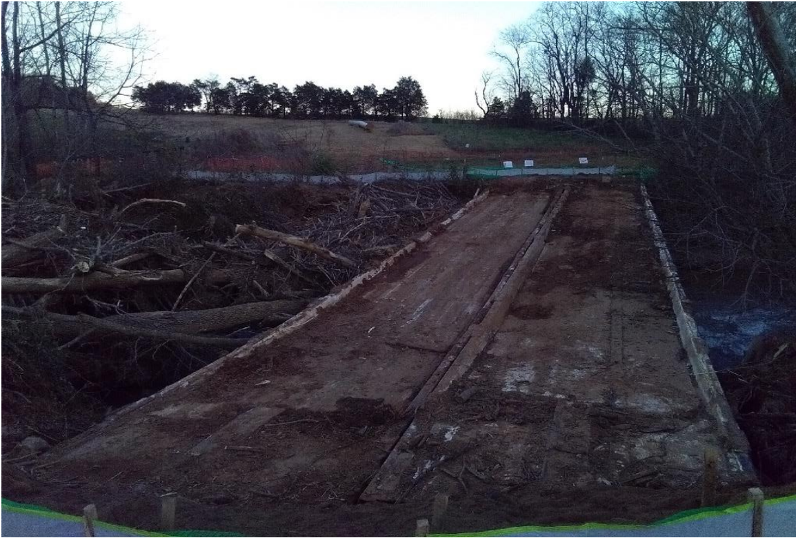
November 13, 2020 Franklin County ground photo shows debris stuck under MVP bridge crossing.
