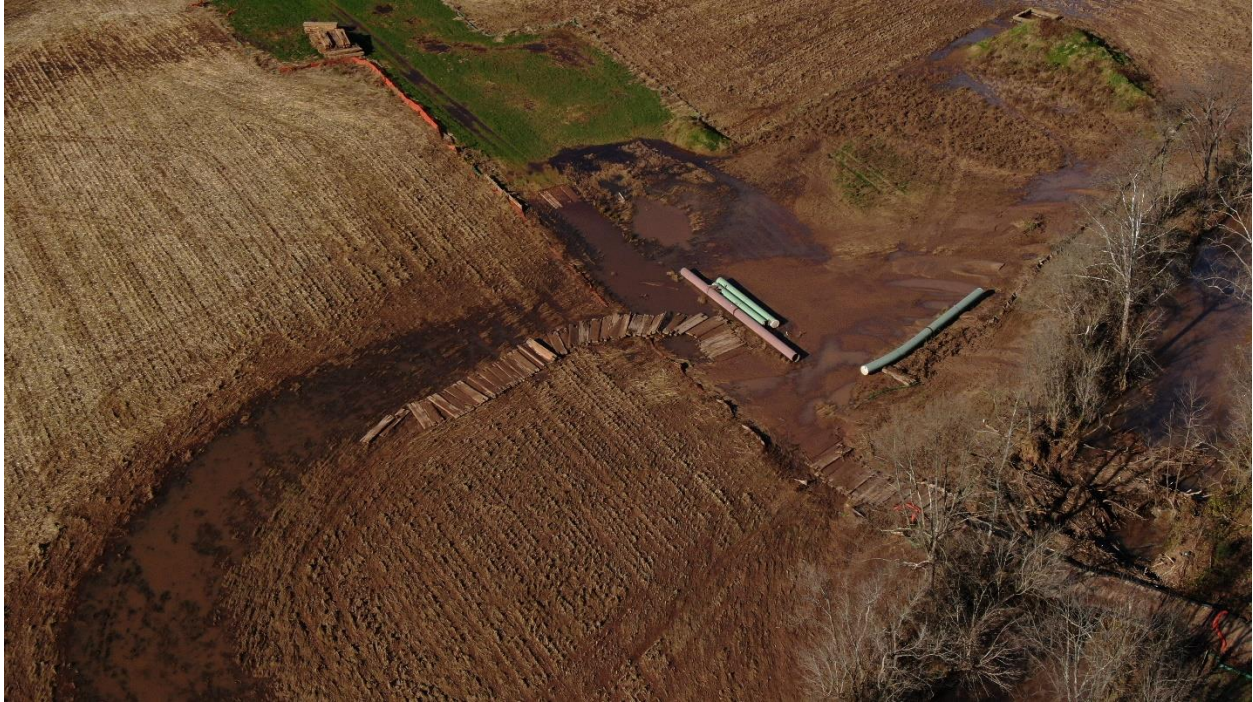
November 13, 2020 Franklin County drone flight shows bridge washout and sediment flowing into stream.
