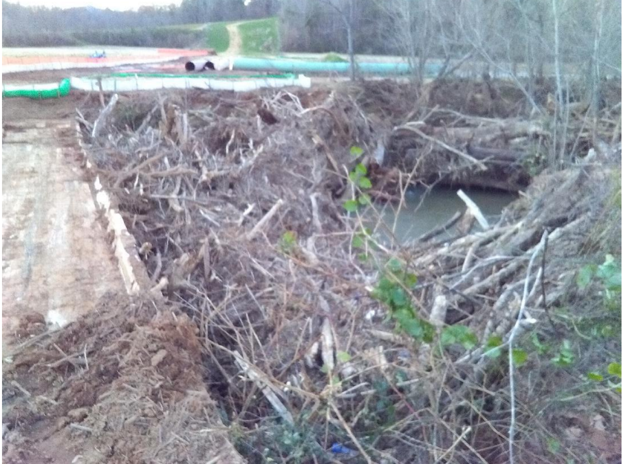
November 13, 2020 Franklin County ground photo shows debris obstructing flow of stream.
