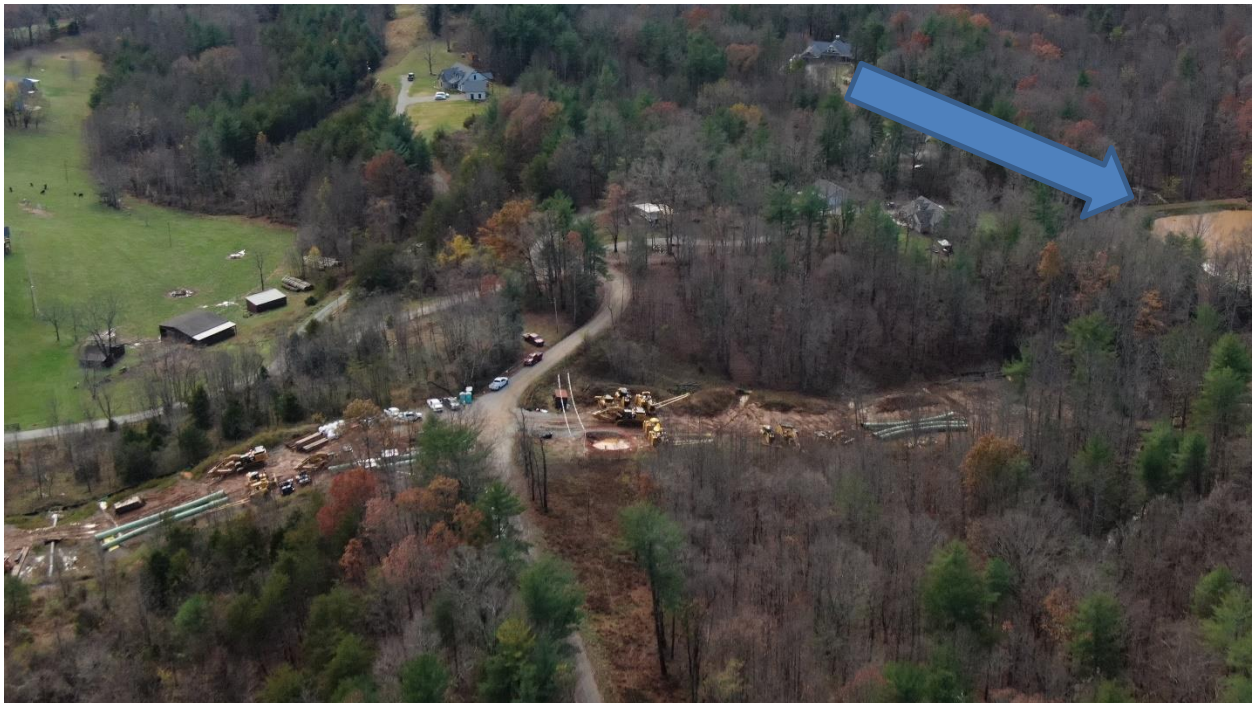
November 13, 2020 Franklin County, Pond below ROW full of sediment.
