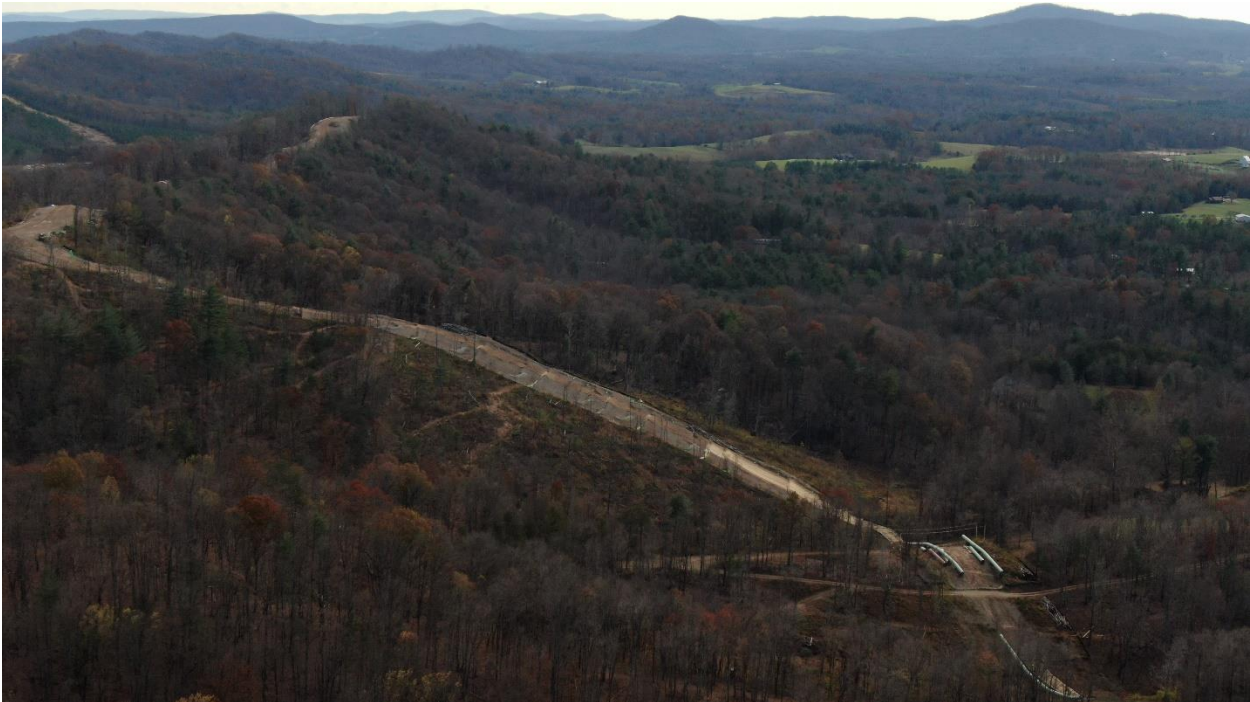
November 13, 2020 Franklin County. Bare areas shown. Jute mesh blanket applied to area eroding at bottom of slope.
