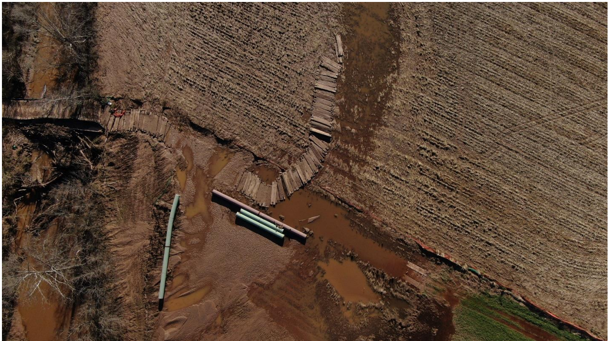
November 13, 2020 Franklin County drone flight shows stream crossing with timber mats displaced by flooding. The stream is brown with sediment flowing from surrounding fields and the MVP right-of-way.
