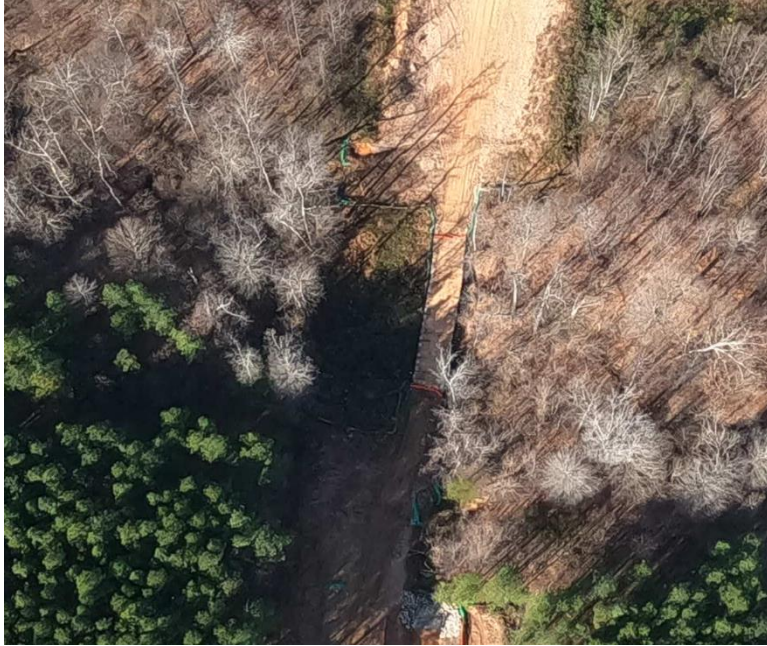
Milepost 294.8 shows evidence of sediment overflowing silt fences and filter socks
