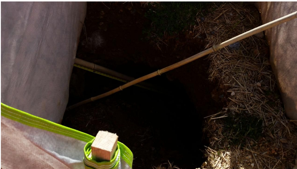
Figure 12: Bottom of the new sinkhole is not visible from the surface.
