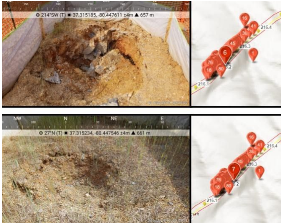
Figure 5: May 2019, two images showing areas of subsidence encircled in silt fence.
