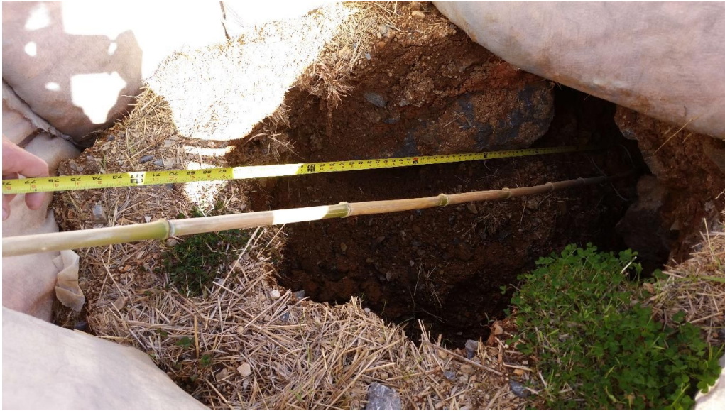
Figure 11: Measurements show the depth of the sinkhole is over 6 feet.
