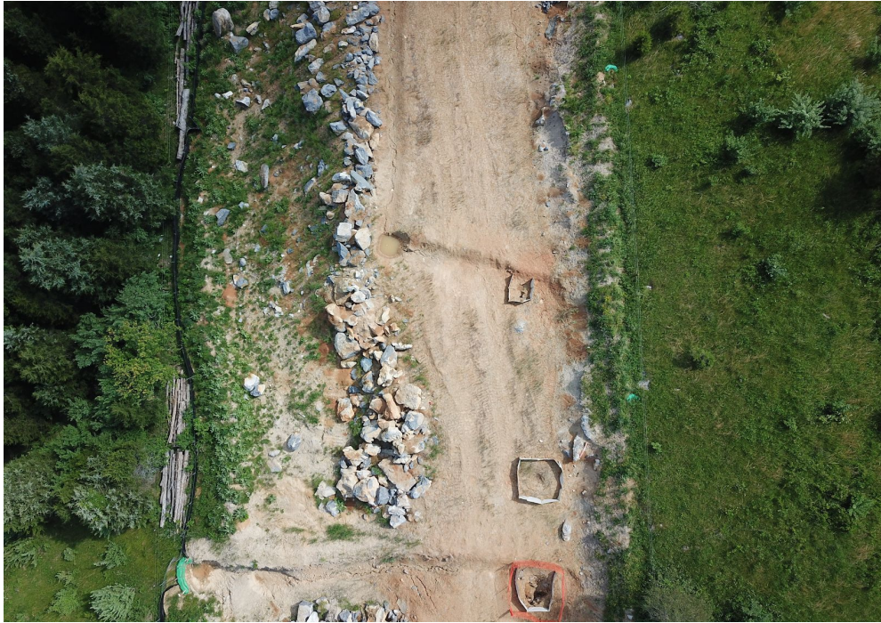
Figure 9: Drone flight photos showing locations of three sinkholes encircled with safety fence in June 2019.
