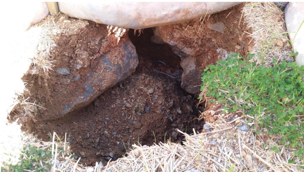
Figure 10: New sinkhole forming in right-of-way on top of the pipeline in the same area shown in Figure 9. Photo taken April 2020.
