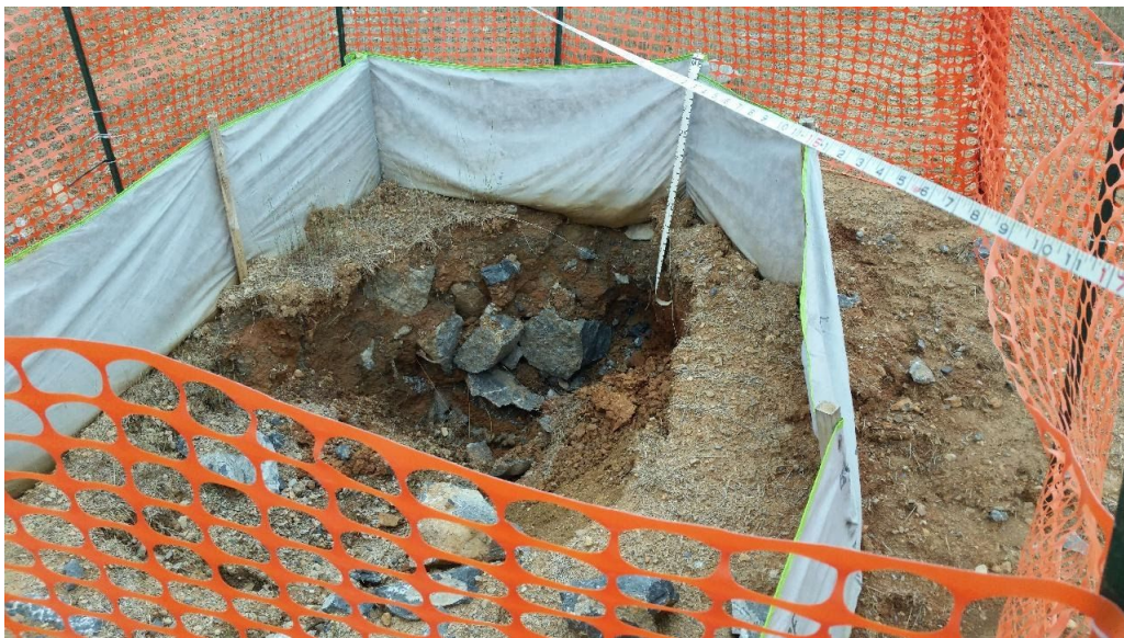
Figure 8: June 2019 site visit shows expanding subsidence.
