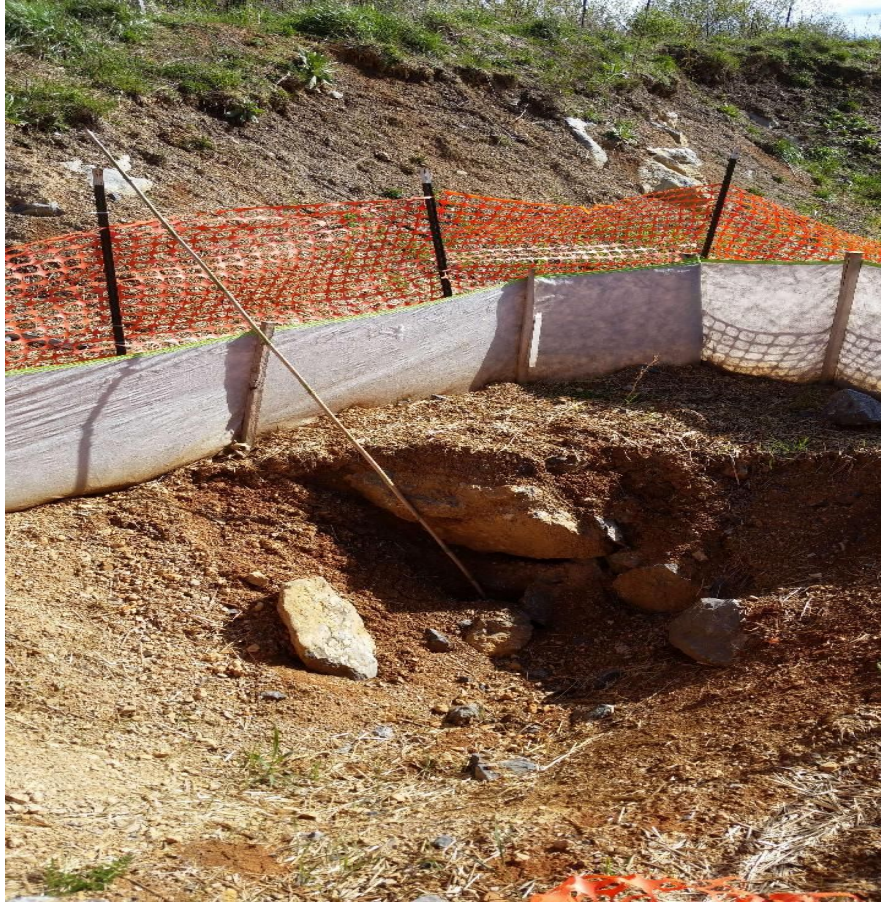
Figure 15: Photo shows sinkhole is continuing to expand.
