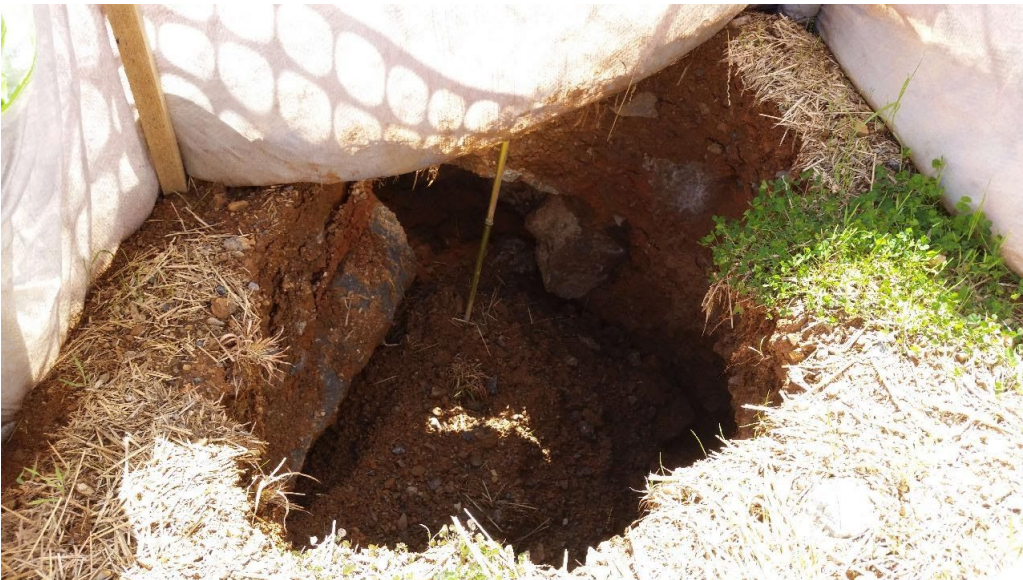
Figure 14: Sinkhole extends into subsurface voids.
