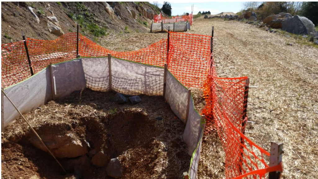
Figure 16: This photo shows locations of four sinkholes within right-of-way. These sinkholes are located adjacent to or over top of the pipeline.
