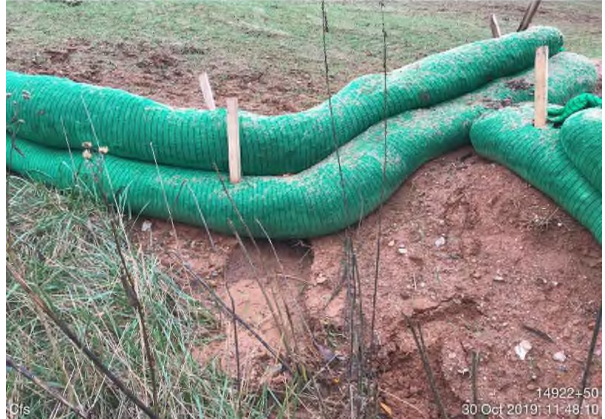
CFS end-treatment bypassed. Maintenance needed. Waterbar lower than CFS outlet.
