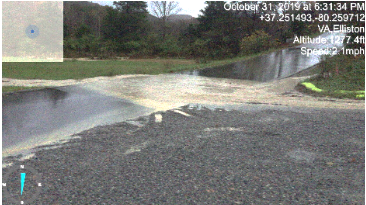
Figure 13: Sediment-laden water leaving MVP's ROW, crossing Bradshaw Road, and entering Bradshaw Creek.
