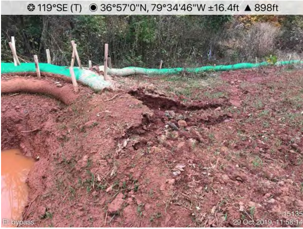
STA 15135+00 CFS end-treatment bypassed. Waterbar lower than CFS outlet.
