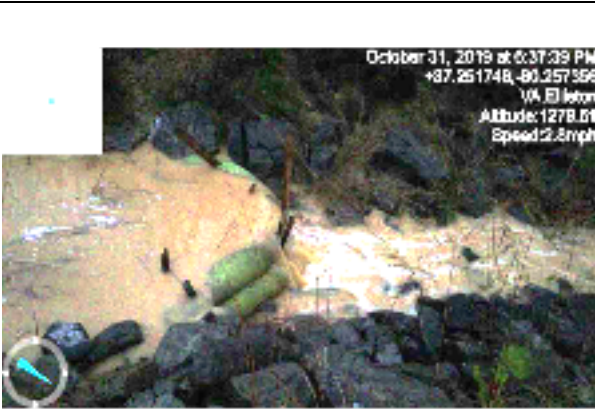
Filter socks overwhelmed by runoff. Drainage area too large for filter socks.
