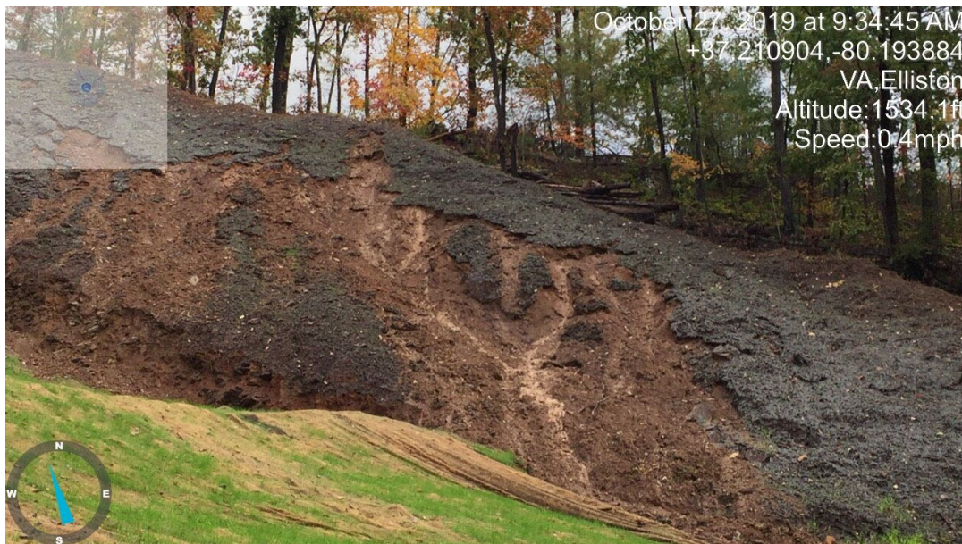
Figure 8: Rill and gully erosion occurring on steep cut slopes
