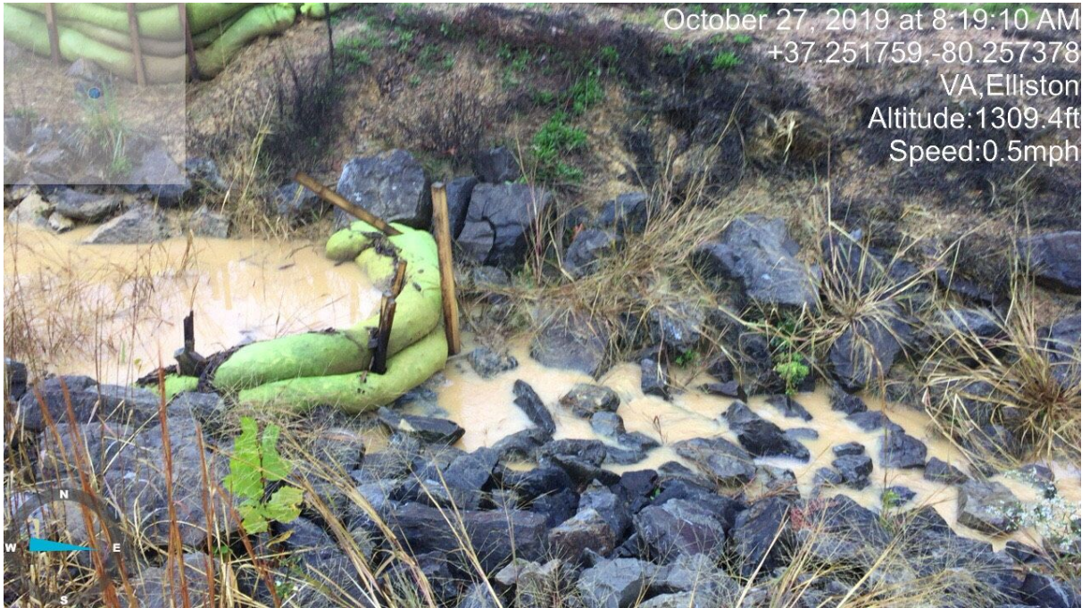
Figure 5: Silt socks overwhelmed by sediment laden runoff flowing off site
