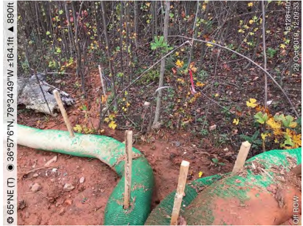
STA 15128+40 Sediment off ROW due to upslope control failure and incorrect installation of waterbar end treatments.
