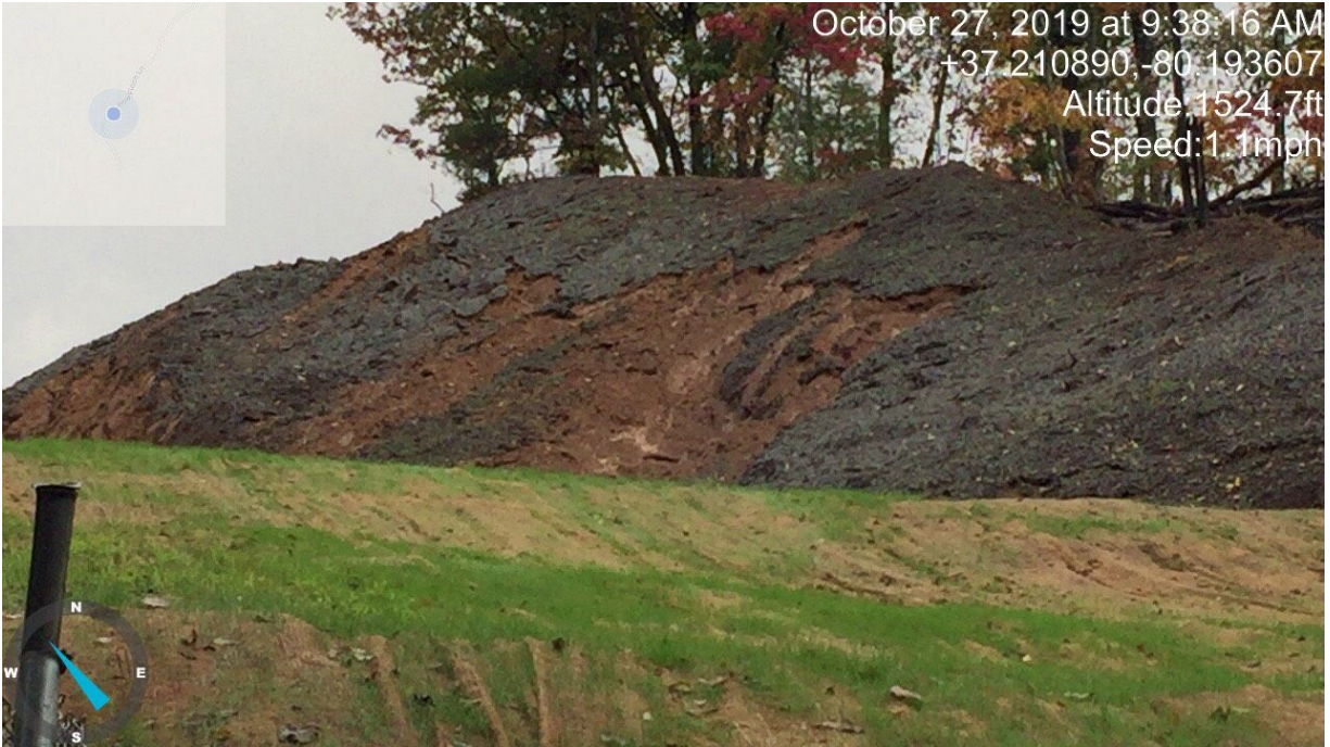
Figure 9: Bare cut slopes forming gullies due to rainfall impact erosion
