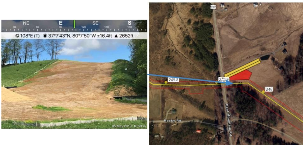
Figure 12: Slope adjacent to Route 221 North still not growing grass.
