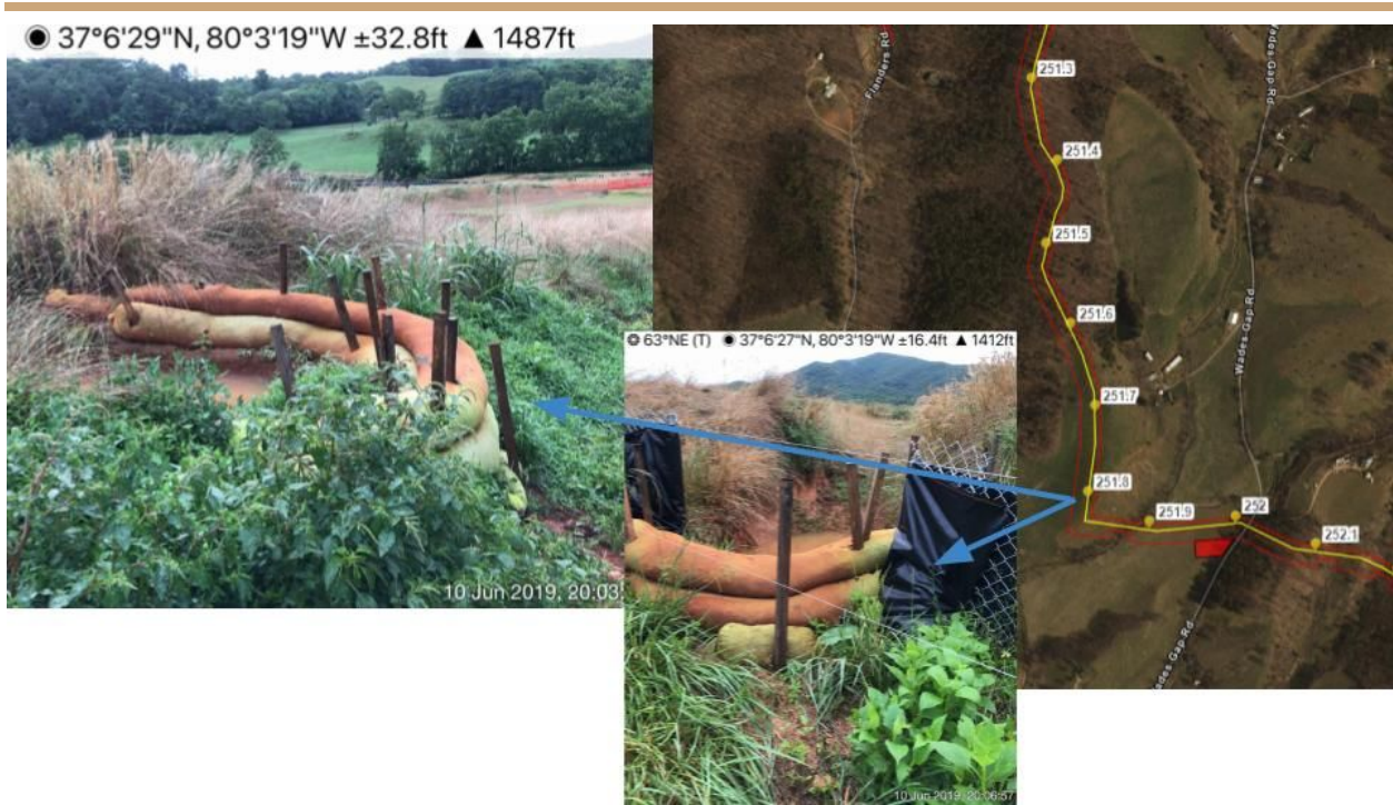
Figure 4: Filter socks overwhelmed by sediment near Wades Gap Road.
