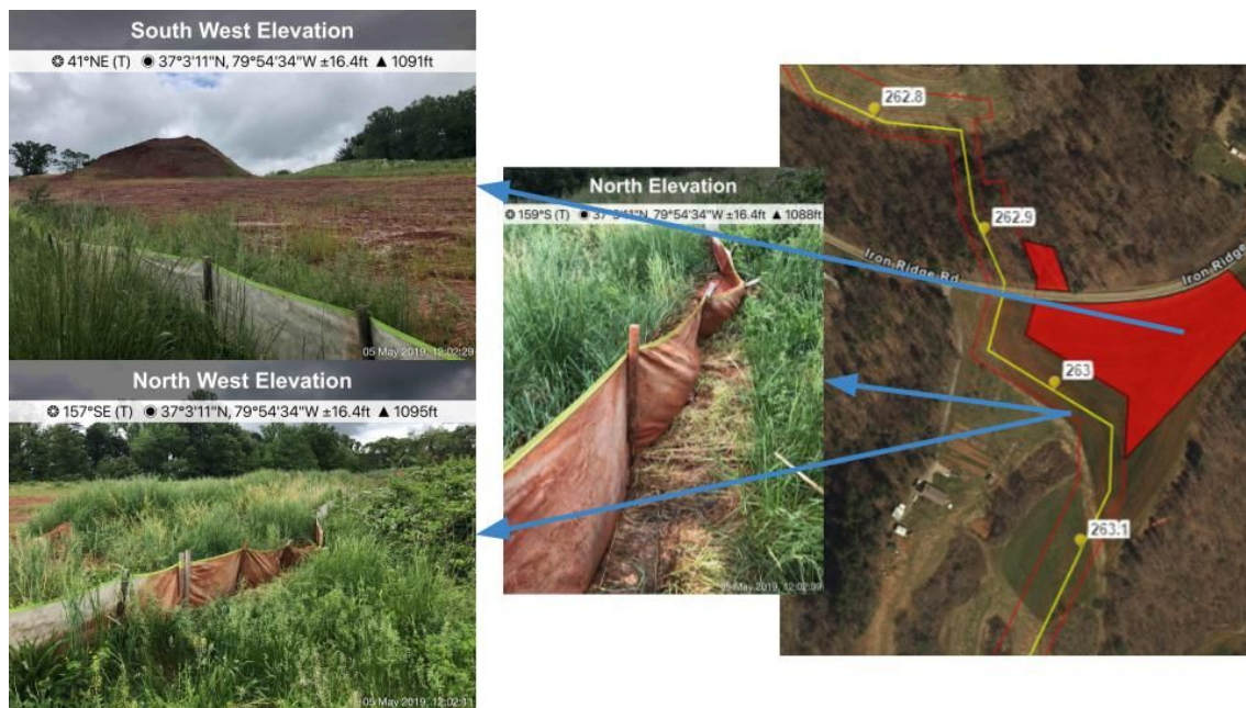
Figure 6: Large stockpile, bare soil, and damaged silt fence on Angle property in Franklin county. (5/5/2019)
