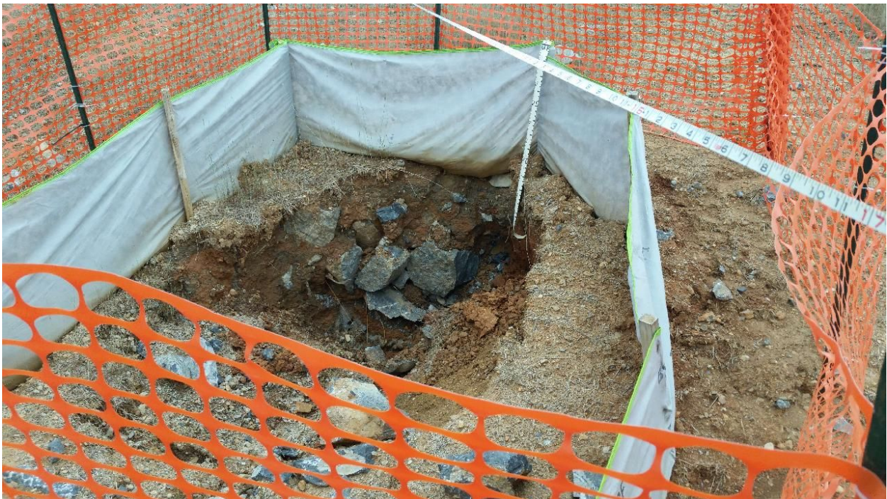
Figure 11: June site visit shows expanding subsidence.
