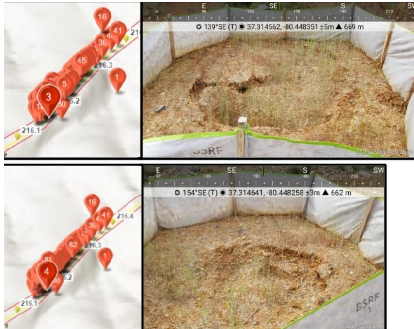
Figure 4: Two images showing areas of subsidence, both are encircled in silt fence.
