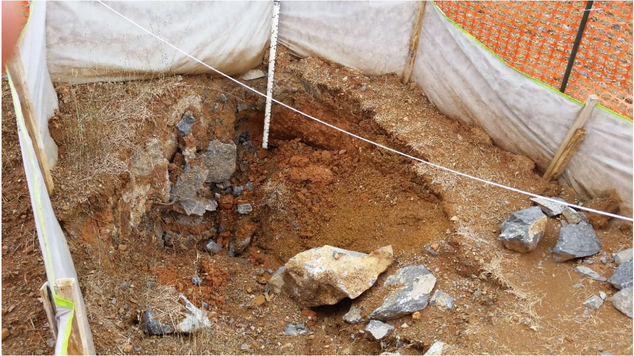
Figure 12: June site visit shows expanding subsidence.
