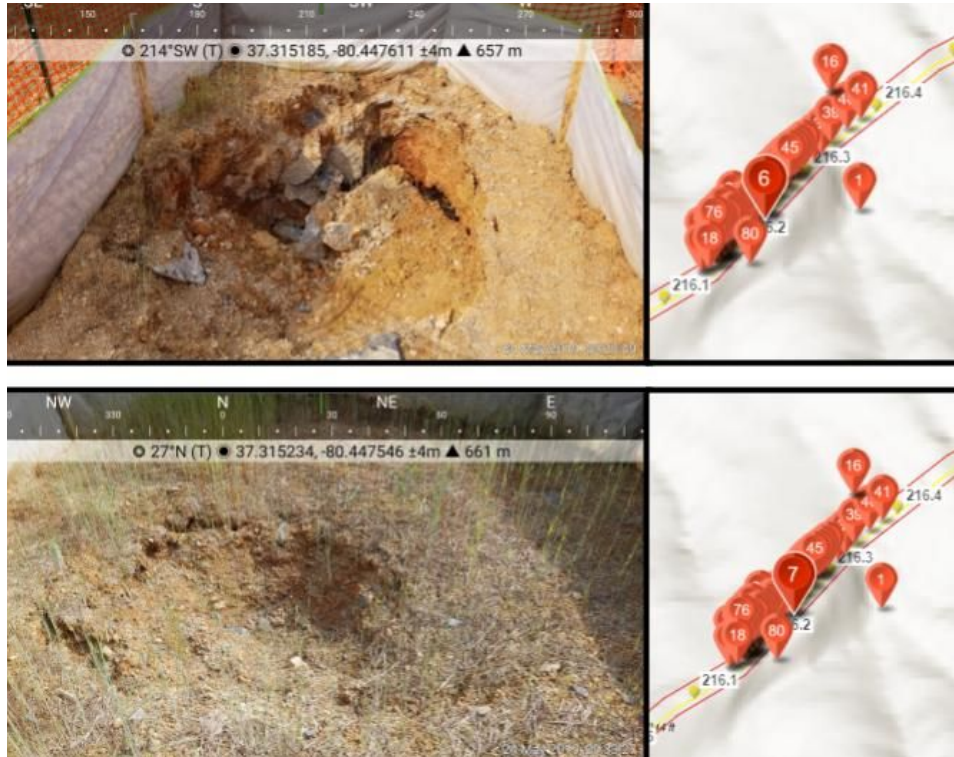
Figure 3: Two images showing areas of subsidence, the top is encircled in silt fence.
