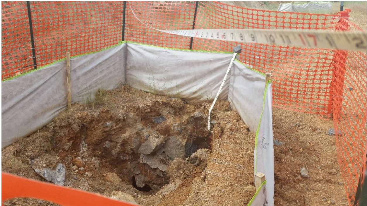
Figure 9: June site visit shows expanding subsidence.
