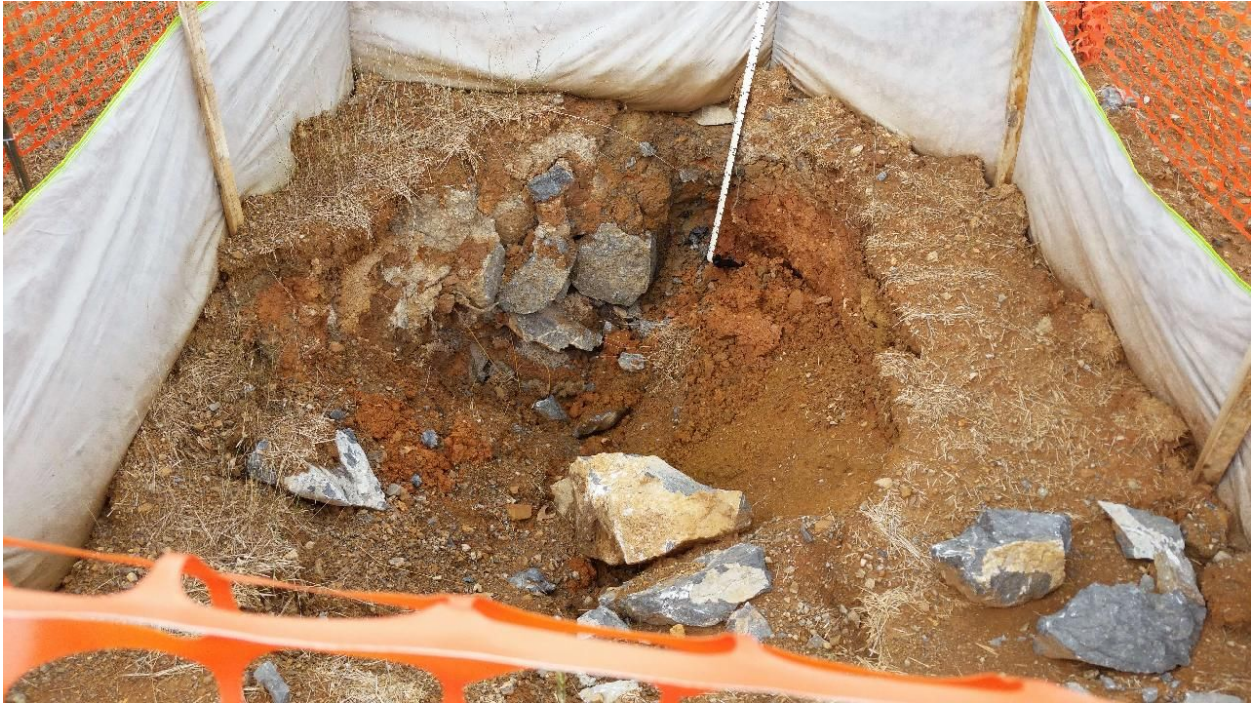
Figure 10: June site visit shows expanding subsidence.
