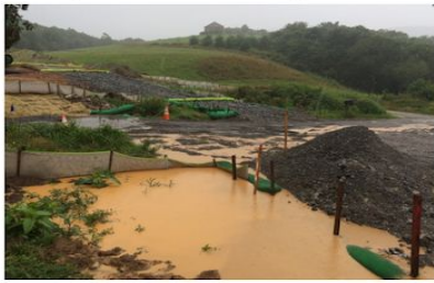
Ineffective silt fence and mulch socks allowing sediment to move into SGT.
