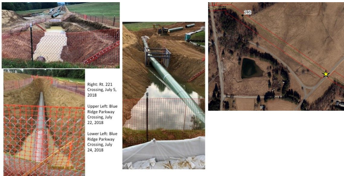
Figure 20: Images from Rt. 221 and Blue Ridge Parkway crossings in Roanoke County in July 2018
