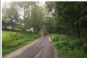
This is 05 Aug at 13:15 hr Friday. After crew departure, a gravel truck arrives and delivers a last load of gravel to the worksite. Note that the road is still receiving copious amounts of sediment and they enter the stream at the damaged streambank.
