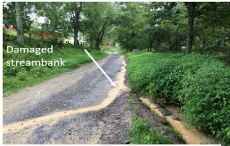
D. The ditch and culvert are still not stopping sediment flow down SGT. This photo at 7:12 am 05 Aug, over 24 hr after last significant rain on Thur , and before MVP Crews begin "cleanup". Why the strange diversion? This is where MVP traffic destroyed the stream bank.
