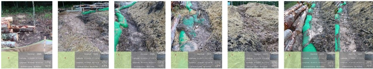
Figure 27: Photos from June 22, 2018 reported incidents on Slayton property
