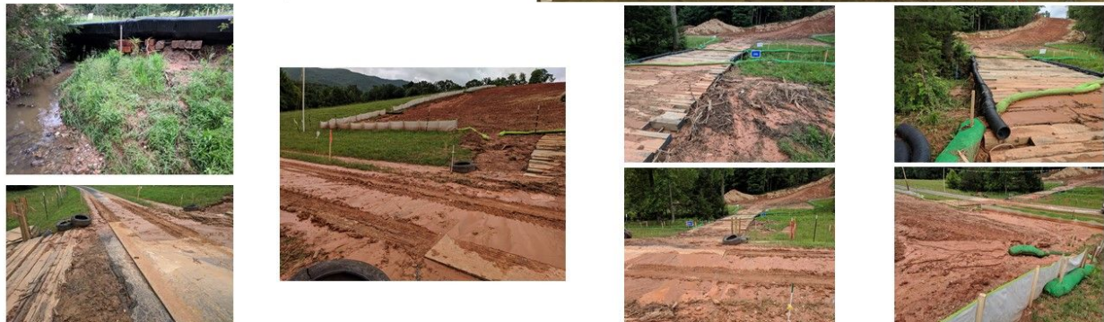
Figure 17: Potential violations reported May 28, 2018
