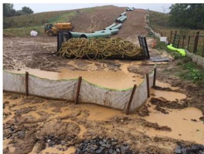
Silt fence in photo failed and has been “reconstructed”, but still actively failing. Standing in approximate centerline, looking eastward toward highly sloping double bench system, and away from SGT.
