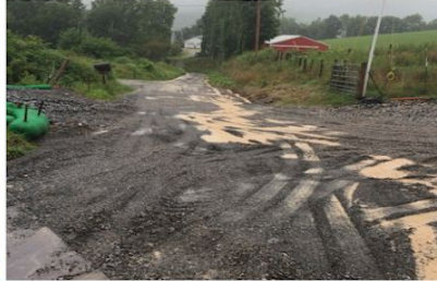
Ineffective gravel placement – now protecting stream crossing to left, but sediment is being channeled to the right side of the road into a recently dug ditch to move it offsite. No BMPs in place here to reduce sediment load within the ditch
