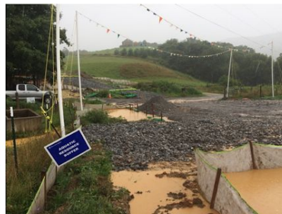
Looking westward toward SGT. Failed mulch socks and silt fencing. Note thick gravel layer placed to fill and hide pooling mud between silt fence and SGT, is not effective in slowing sediment loss. Besides BMP failure, sediments are clearly entering 1) an Aquatic Resource Buffer, 2) a State Road, 3) a
