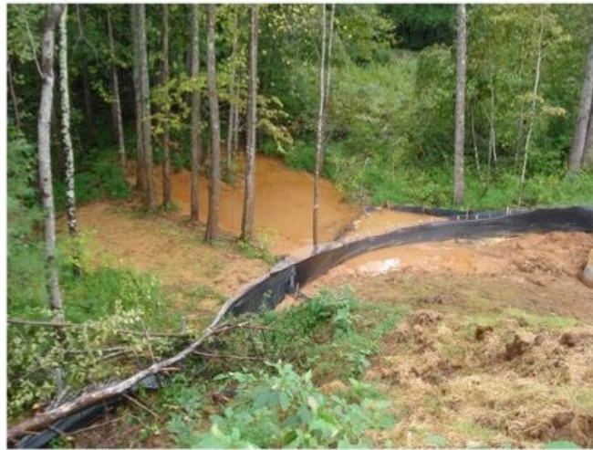
Figure 3: Large amount of mud streaming off of site at Cahas Mountain Road Crossing, despite perimeter controls in place. September 17, 2018.
