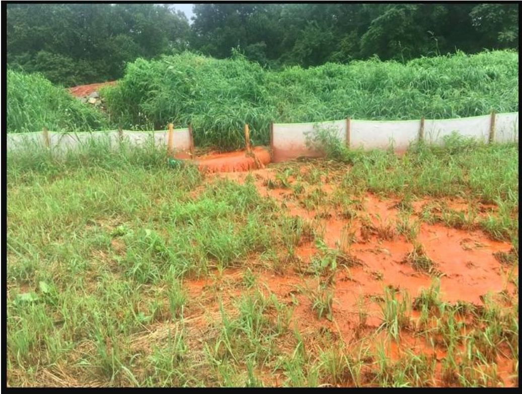
An example of failure of an outlet protection structure. Angle Property, August 3, 2018 (outlet from water bar failing).
