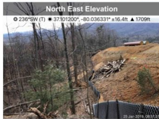
Figure 10: Construction on the ridge of Cahas Mountain, unsecured earth above numbered stream crossing on January 25.
