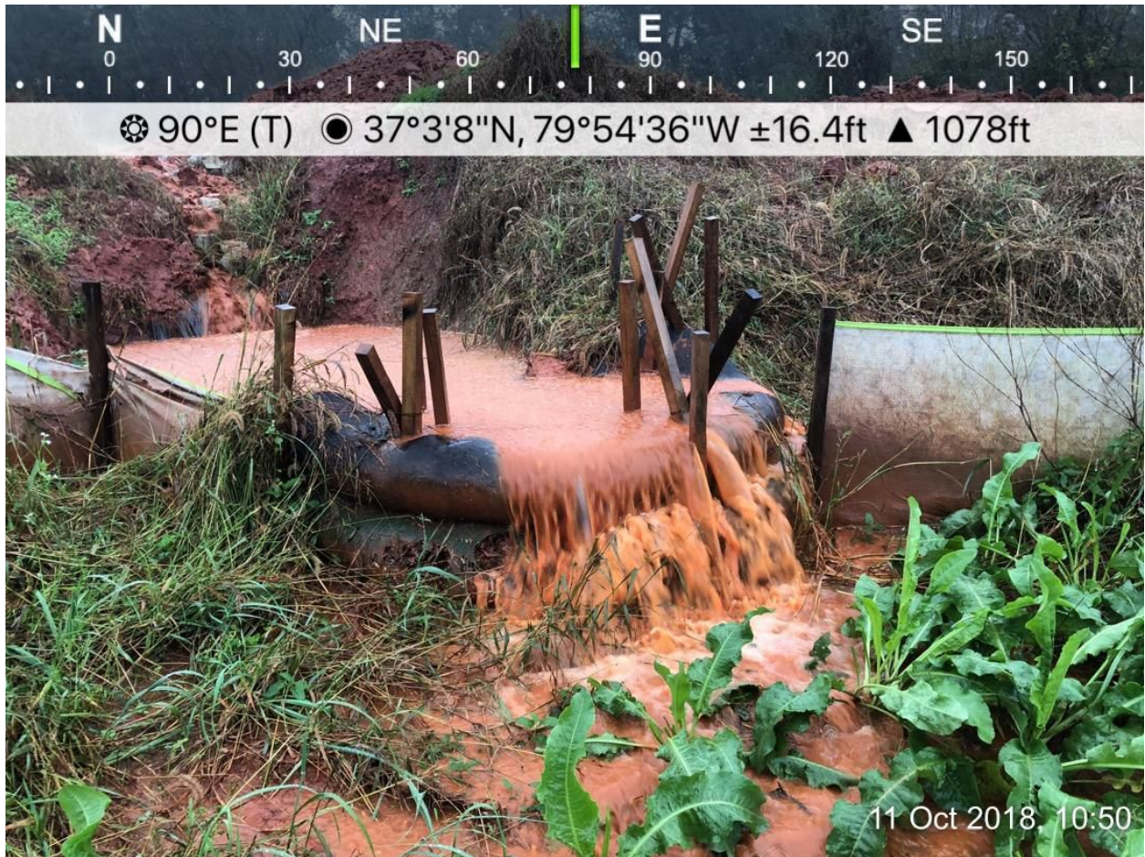
Outlet structure failure. Angle property, October 11, 2018
